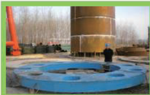
Annular load cell for caisson
